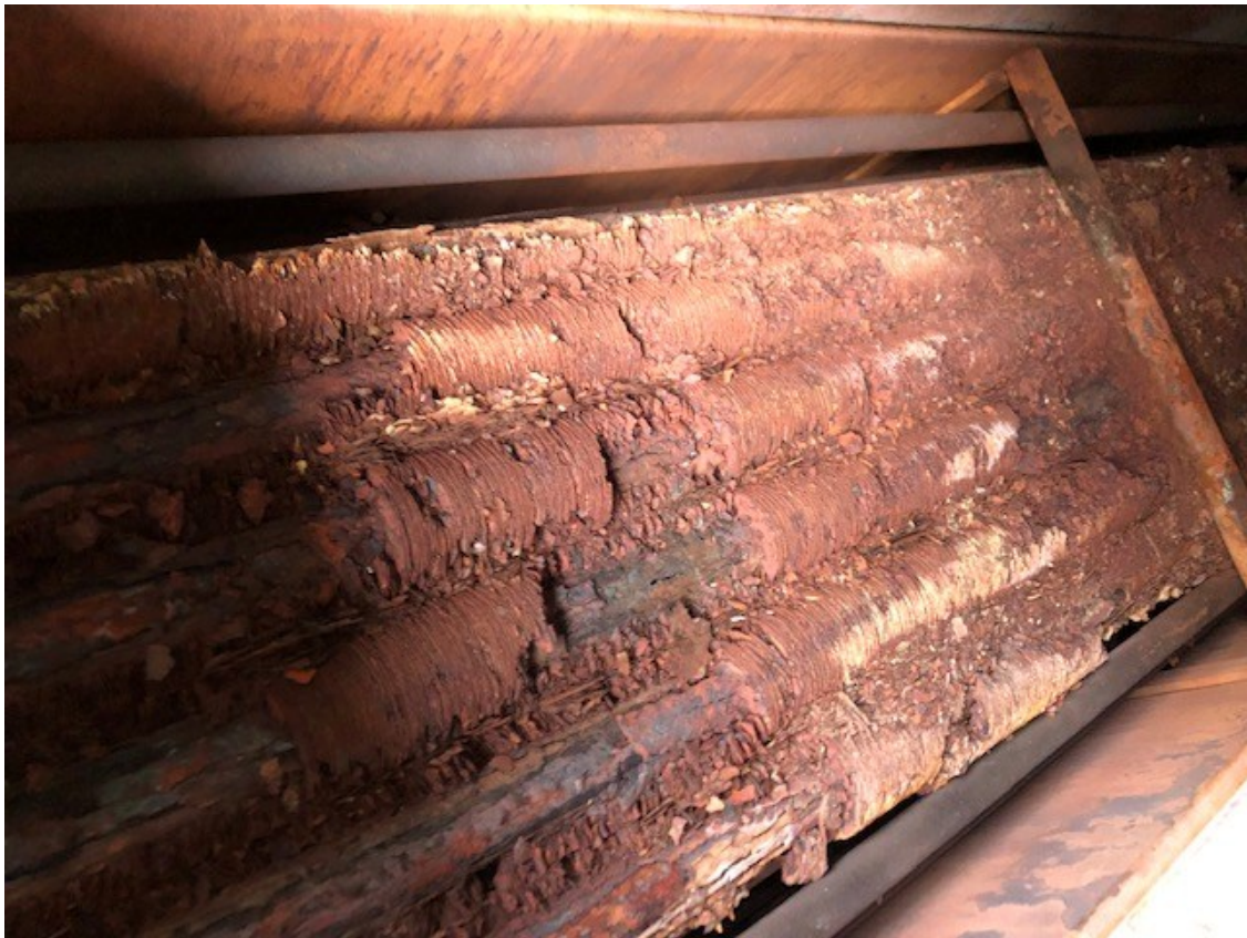
Figure 5.13: Condensation damage after months of operation on a finned tube heat exchanger that worked in unintended condensing operation.
