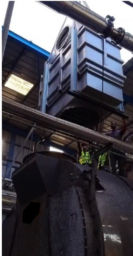
Figure 5.12: The PPHE shown in Figure 5.9, inside its frame, during mounting on 20.000t/h steam boiler.
