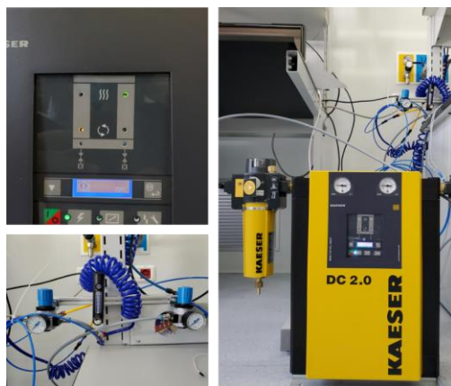
Fig. 7.16: (Right) Kaeser DC2.0 dryer unit, (left-up) dewpoint set to -70^{\circ}\text{C} , (left-bottom) flow meter.
