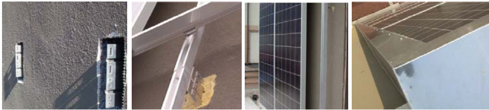
Figure 5.3: mounting system of the modules integrated in the Ex Post building façade [source: Elpo]
