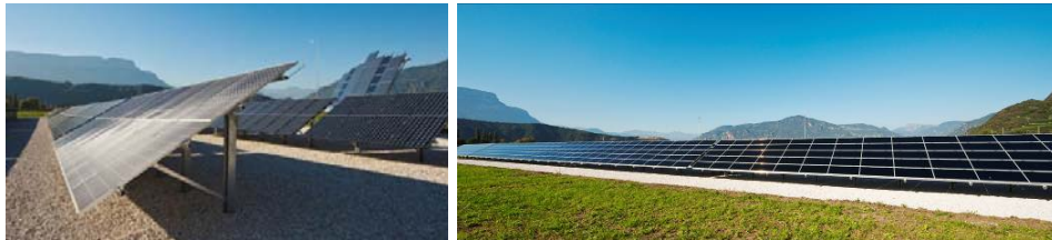
Figure 5.8: ABD PV Plant. Experimental plant on the left and commercial part on right
