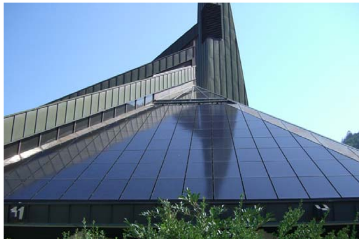
Figure 5.5: Picture of the roof integrated PV system of the Milland Church in Bressanone (North of Italy)
