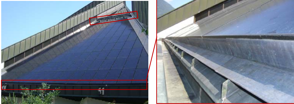
Figure 5.6: On the left: picture of the BiPV system highlighting the inlet and outlet air gap sections. On the right: zoom which shows the reduced air gap section
