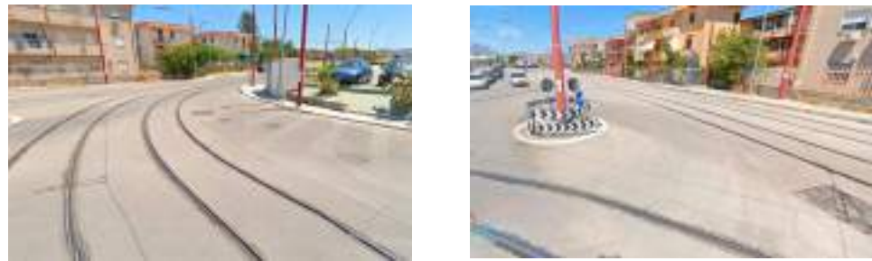
Figure 24. Photos of the analysed road pavement (via Carlo Guli)—class B tramway line.
