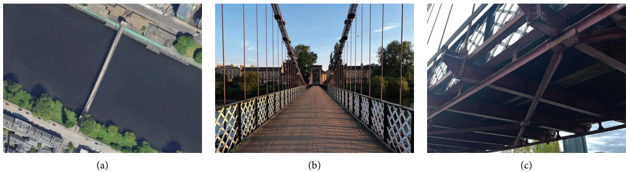
FIGURE 7: Overview and structural details of the bridge: (a) aerial view of the bridge; (b) view along the top of the bridge deck; (c) view of the underside of the steel truss deck structure.
