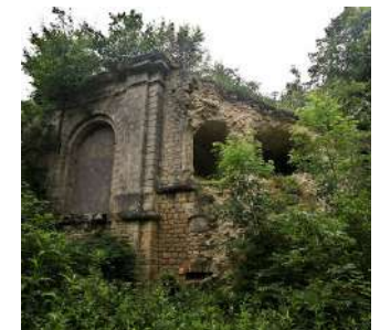
Du Rozelier Fort Destruction -State of abandonment
