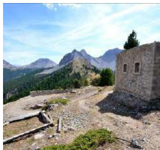
Fort Lauzette State of abandonment
