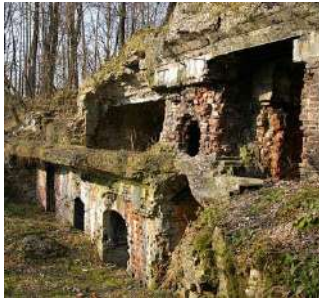
Krakow - Fort 74 1/2 State of abandonment
