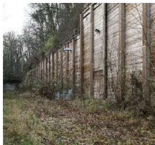
Fort Kameke State of abandonment
