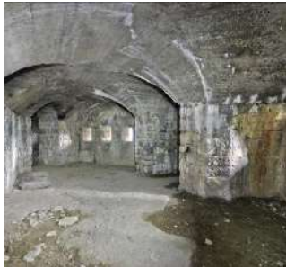
Fort Truc State of abandonment
