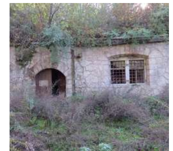
San Rocco Fort State of abandonment
