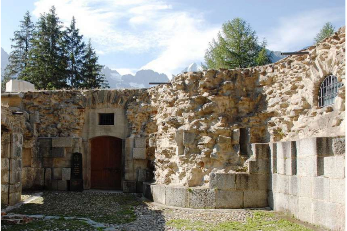
Pic.7.2 Fort Strino, detail of cladding in worked blocks and core with sharp-edged stones.
