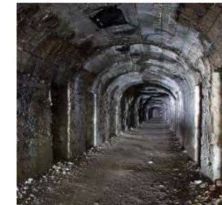
Monte Orsa Fortified position State of abandonment
