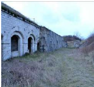
Fort de Domgermain State of abandonment
