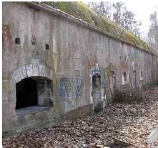
Fort Tarpno State of abandonment
