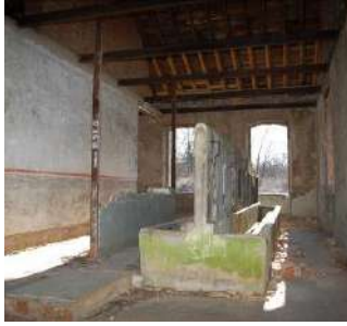
Ouvrage de Chevremont State of abandonment
