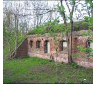
Krakow - Fort 49 1/2 State of abandonment
