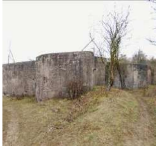
Ouvrage de Francheville State of abandonment
