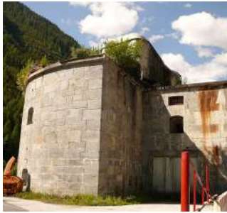
Fort Gomagoi State of abandonment
