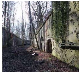
Fort de Dave - Namur State of abandonment
