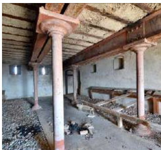
Fort Grand Maye State of abandonment
