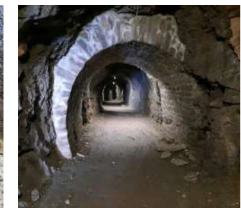
Monte Morissolo Cavern State of abandonment
