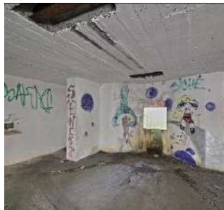
Fort du Chanot State of abandonment
