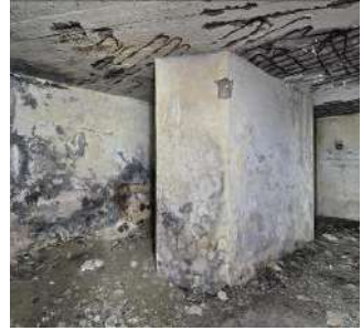
Ouvrage de Charmes la Cote State of abandonment
