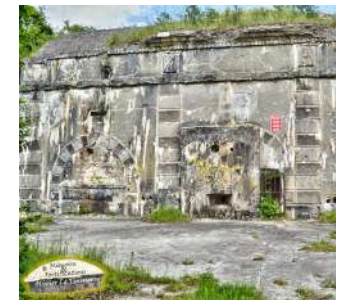
Moulainville Fort State of abandonment
