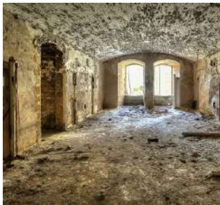
Fort St. Julien State of abandonment
