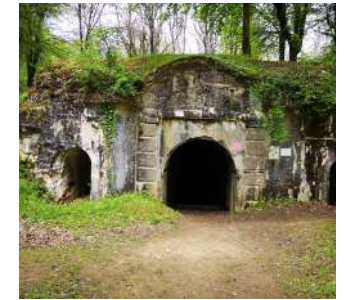
Sauville Fort State of abandonment
