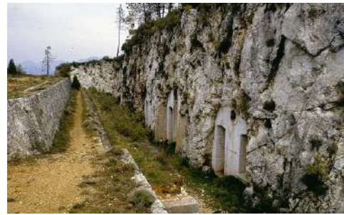
Mont-Chauve de Tourette Fort State of abandonment
