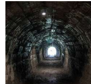
Monte Morissolo Cavern State of abandonment
