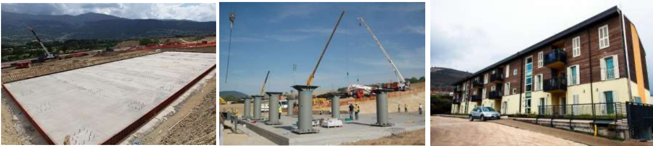
Figure 21 - Progetto C.A.S.E. . Concrete slab, anti-seismic system and finished flat – source: Cosimo Colizia and Paolo Marronaro [63]
