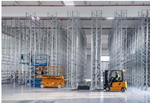
Fig. 1. A typical steel storage rack (courtesy of Metalsistem S.p.A.).
