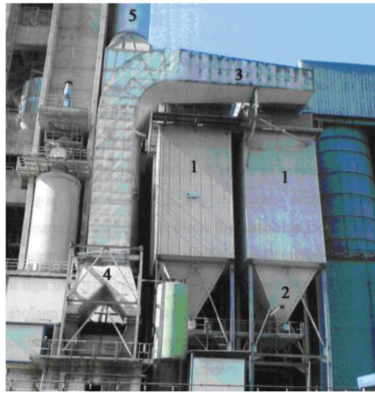
Figure 1: Sketch of the case study hybrid collector. (1) Final sections of the fabric filters; (2) hoppers; (3) de-dusted air duct; (4) fan; (5) bottom of the chimney. The ESPs are located behind the fabric filters.
