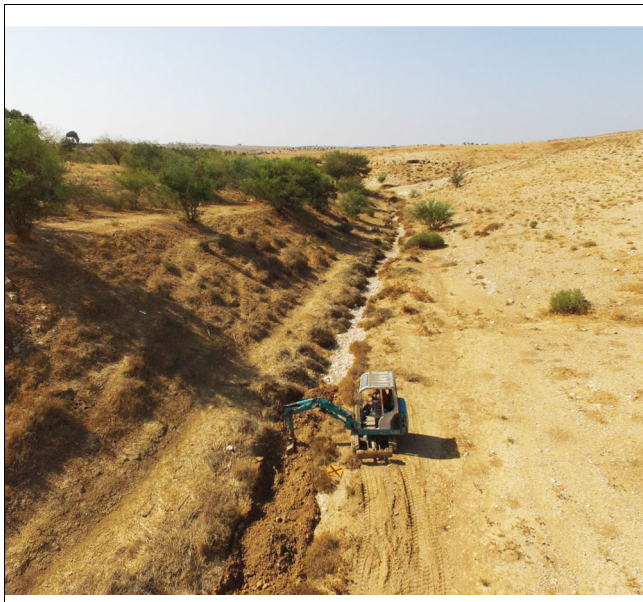
FIGURE 4 Downstream view of the Yatir study reach as a mini excavator was mixing the channel bed material, thereby destroying the sedimentary and topographic character of the flat-bar sequence.
