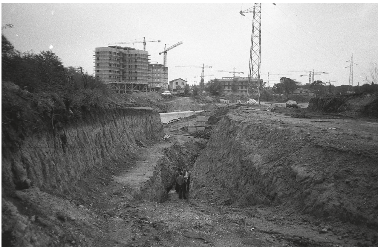
Fig. 13 - Digging trench of the sewer collector at Casal de' Pazzi: researchers observe levels with fossils.
