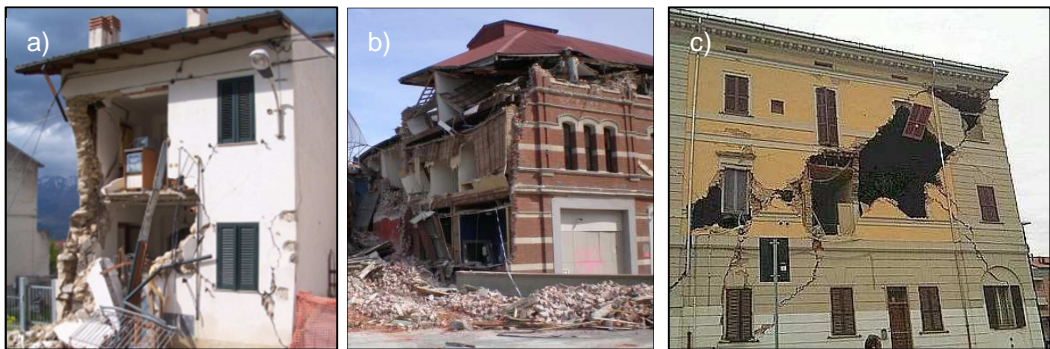
Fig. 1.1 Out-of plane failure of masonry walls: a) L'Aquila Earthquake, Italy (2009) [Bursi et al. (2009)]; b) Christchurch Earthquake, New Zealand (2011) [Dizhur (2011)]; Emilia, Italy Earthquake (2012) [www.adnkronos.com].
