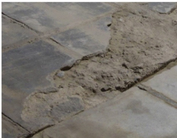
Fig. 5. Frost heaving damage on a concrete structure (reprinted from Ref. [77]).
