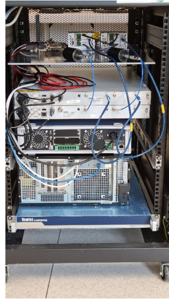
(b) Transponders rack
