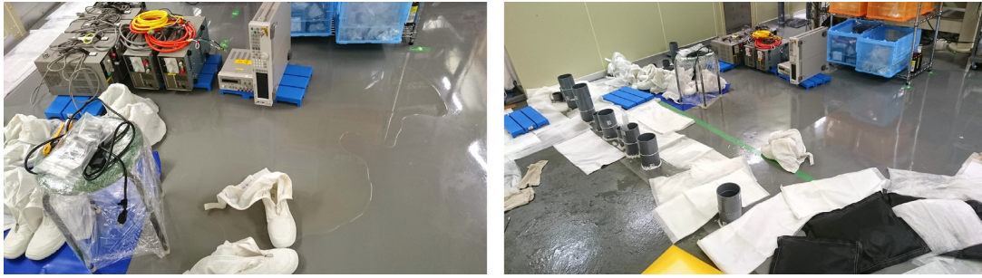
Fig. 3. Spring water leaking on the floor in the PSL room. (Left) The entire floor of the room was wet. (Right) Pipes were placed at the leaking points on the floor to prevent the water from spreading further. Water-absorbing sheets are also seen. The legs of the optical table can be partially seen on the top right. The photographs were taken in March 2015.
