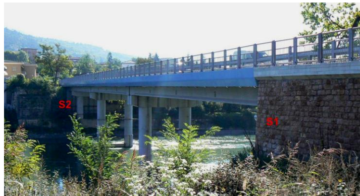
Fig. 2.5 Overview of the SP90 Bridge on the Adige River at Villa Lagarina
