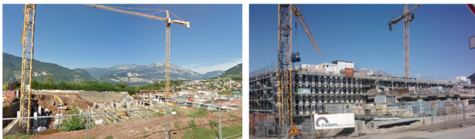
Figure 3.13: New large building in the Trento dataset: some month before the 2011 TerraSAR-X acquisition (on the left) and on the same day of the second acquisition (on the right). As one can notice the building is still under construction during the second acquisition with several materials and vehicles present in the building site.
