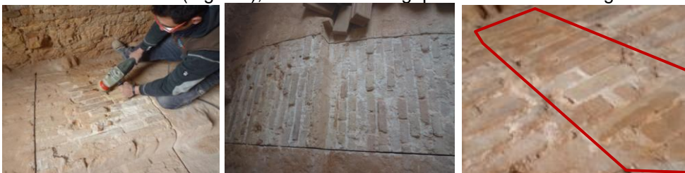
Fig. 5.8 Cleaning and masonry surface, in red, area cleaned for CFRP application (right)
