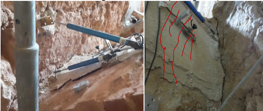
Fig. 5.57 Debonding and diffusion of cracks in the anchorage on A (load side)
