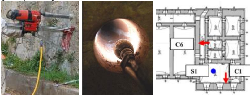
Fig. 4.9 Coring machine (left) and video endoscopy(centre), test on the East tower (right)
