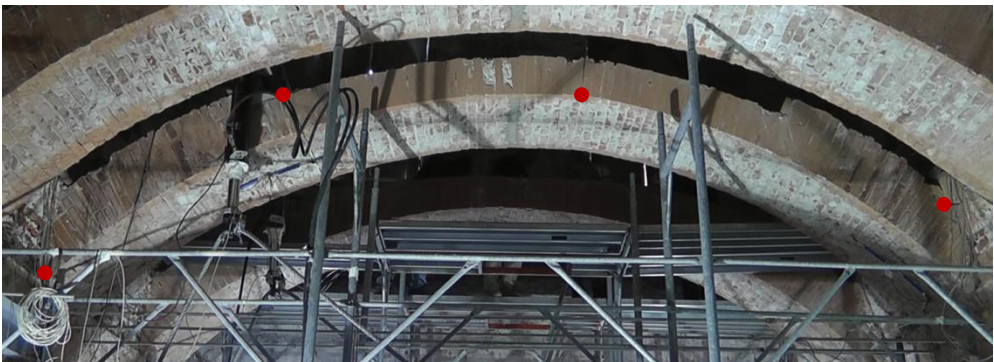
Fig. 5.33 Unreinforced vault at moment of maximum load application
