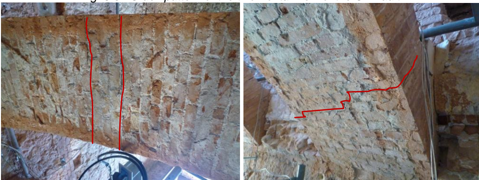
Fig. 5.35 Cracks in the Intrados hinges, B on the left and D on the right
