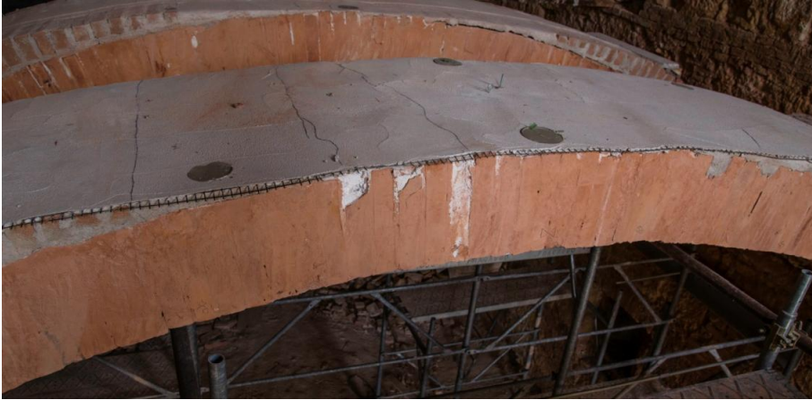
Fig. 5.68 Crack diffusion in the textile reinforced mortar
