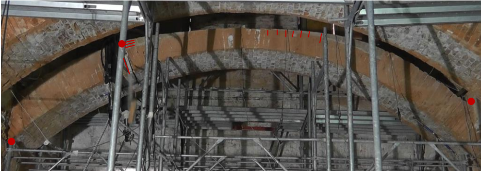
Fig. 5.46 CFRP vault at the highest displacement
