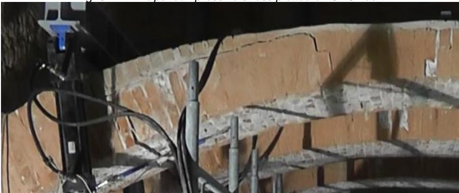
Fig. 6.72 Zoom on the failure
