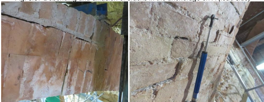
Fig. 5.58 Small sliding of joints under the loading point (left) and near hinge D (right)
