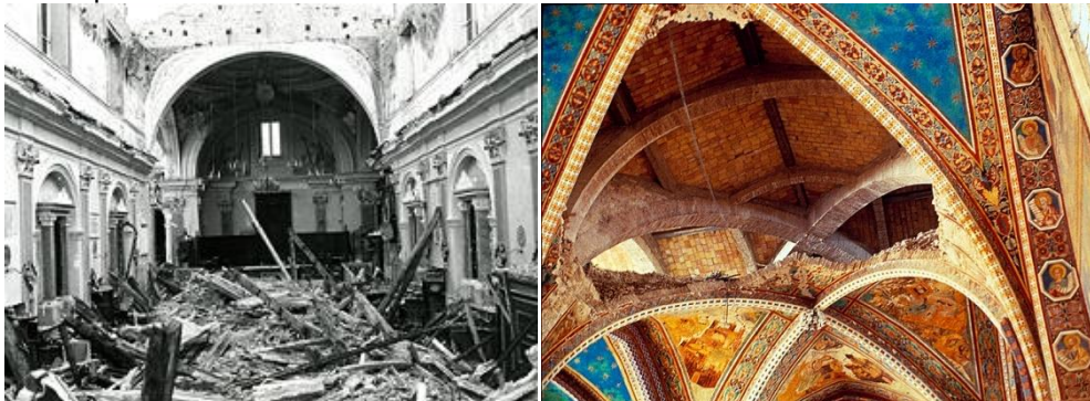
Fig. 2.47 Vault collapsed after Friuli earthquake 1976 (left), S. Francesco d'Assisi vault collapse 1997 (right)
