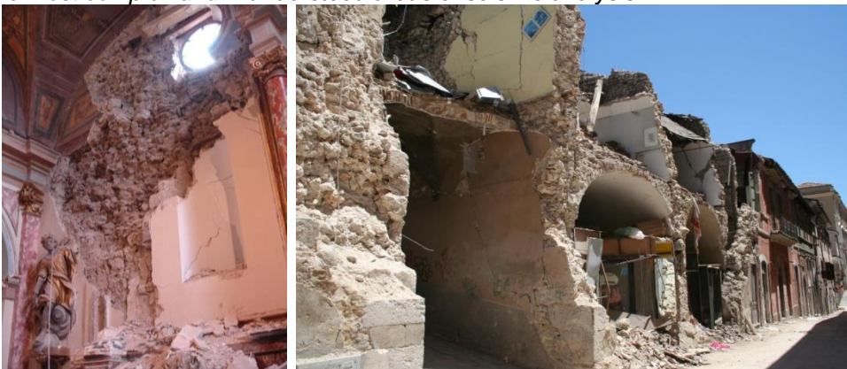
Fig. 2.1 Material failure in San Michele Arcangelo, Celano (left) local collapse, via Arrischia, L'Aquila (right)
