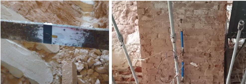
Fig. 5.74 Strain gauge applied on the existing tie (left) and on the setup ties (right)
