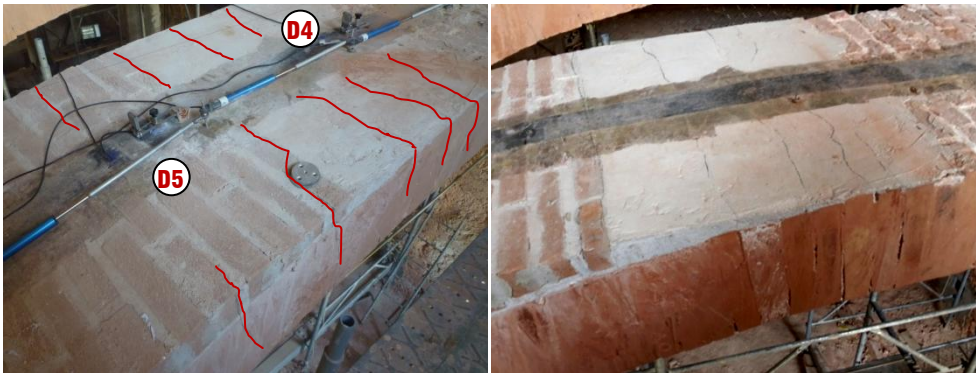
Fig. 5.54 Cracks spreading due to composites application
