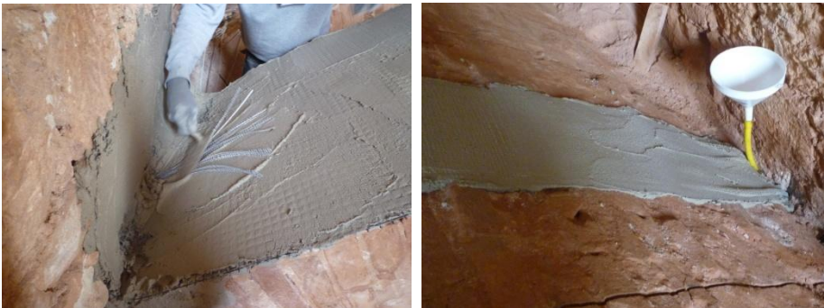
Fig. 5.16 Steel anchorage for the Basalt net and injection of mortar based composites
