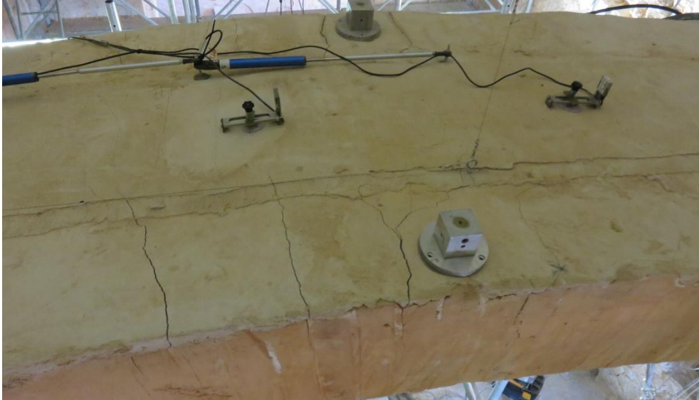
Fig. 5.59 Crack diffusion due to composites action
