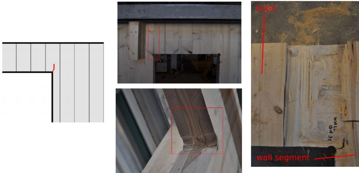
356 357 Figure 9: failure in the lintel of Wall 01 (D_3_S)
