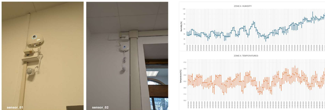
Fig. 60. Indoor sensor deployment and measured environmental data. Left: installed temperature and humidity sensors in the monitored zones. Right: corresponding time series of relative humidity and air temperature used for DT calibration and validation.
