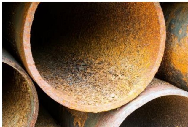
Figure 2 - Pipes damaged by internal corrosion (Source: Mihir S. archive).
