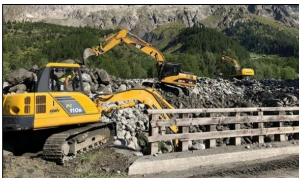
Fig. 2. Mechanical removal of the clogging occurred during the debris flow event of August 2018 in Val Ferret, near Courmayeur (AO, Italy).
