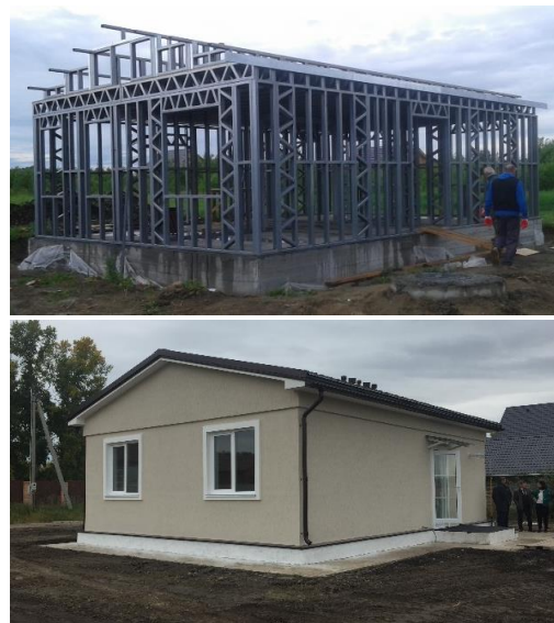
Fig. 1 – The building during (a) and at the end of the construction phase (b). Picture by Giovanni Manzini, 2019
