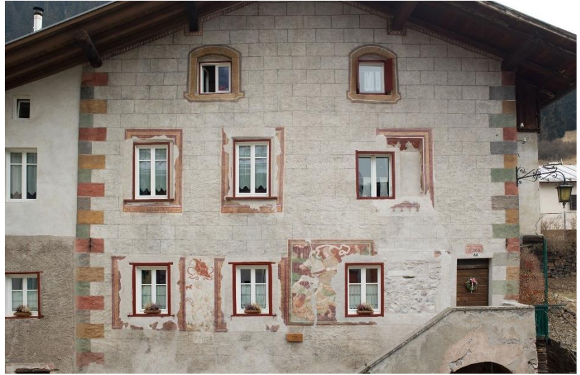
Figure 4.7 - From top to bot- tom: main façade of Casa Tinol, stone wall and survey activities: topographic sur- vey and level plane definition. Images by LA- MARC acquired during the first acquisition phase in September 2021.
