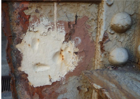
Figure 180. WWII damages + shielding material.
