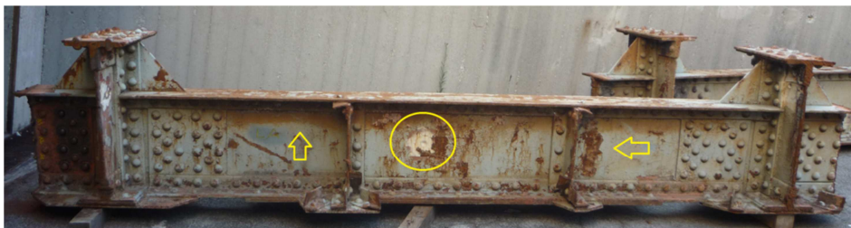
Figure 57. Rail bearer: corrosion and damage.
