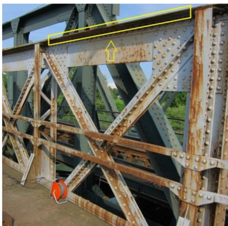
Figure 52 Lateral plates zone.
