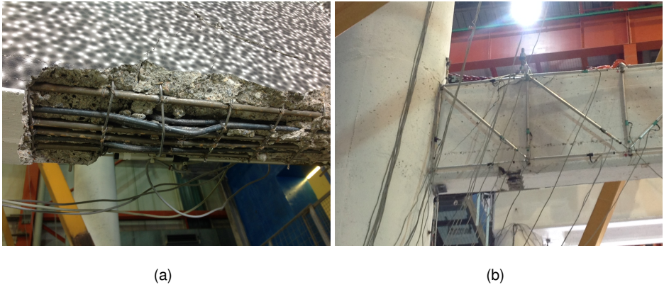
Figure 4.40: a Expulsion of the concrete cover on transverse beam of Pier #11; b crack pattern of the lower transverse beam of Pier #9 after Test k12, i.e. non isolated bridge at ULS 200%.
