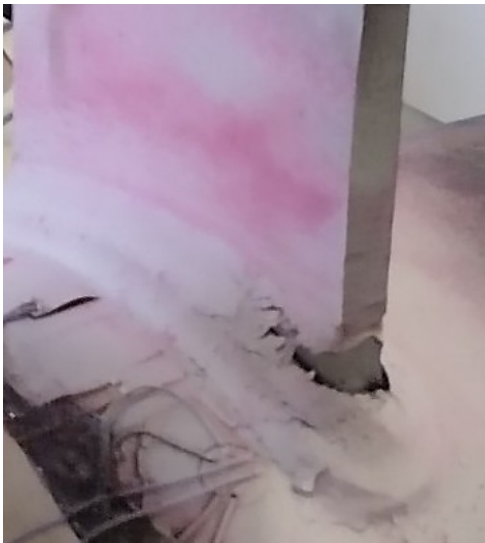
(a) Initiation of failure and stress concentration on the corners
