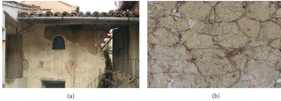
FIGURE 1: (a) Typical raw earth cob architecture at the “Villa Ficana” district of Macerata, Italy; (b) cob elements constituting an existing wall.
