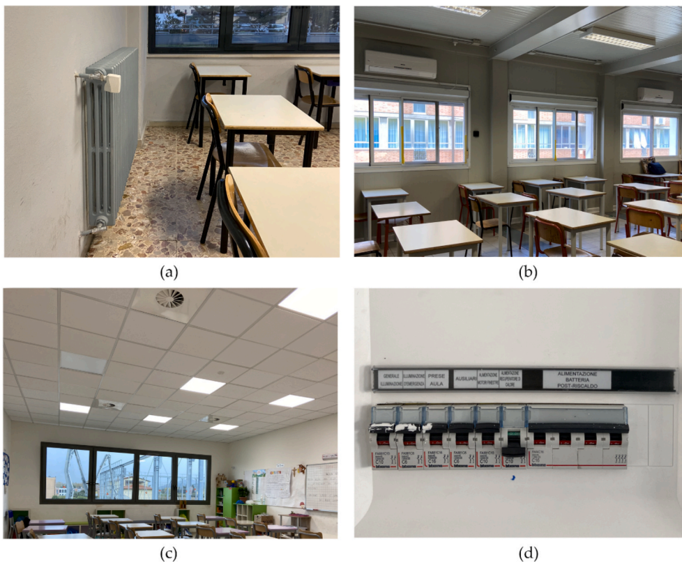
Fig. 1. Examples of different heating and ventilation systems in the surveyed buildings: (a) not controllable central heating system; (b) controllable split air conditioner system; (c) not controllable mechanical ventilation system; (d) controllable mechanical ventilation system: control panel.
