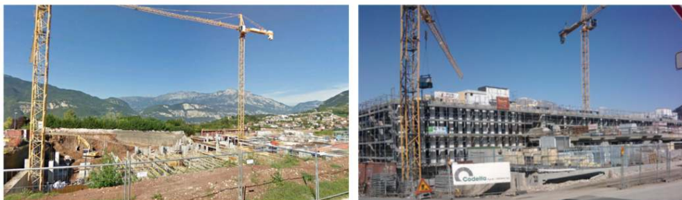
Fig. 14: New large building in the Trento dataset: some month before the 2011 TerraSAR-X acquisition (on the left) and on the same day of the second acquisition (on the right). As one can notice the building is still under construction during the second acquisition with several materials and vehicles present in the building site.
