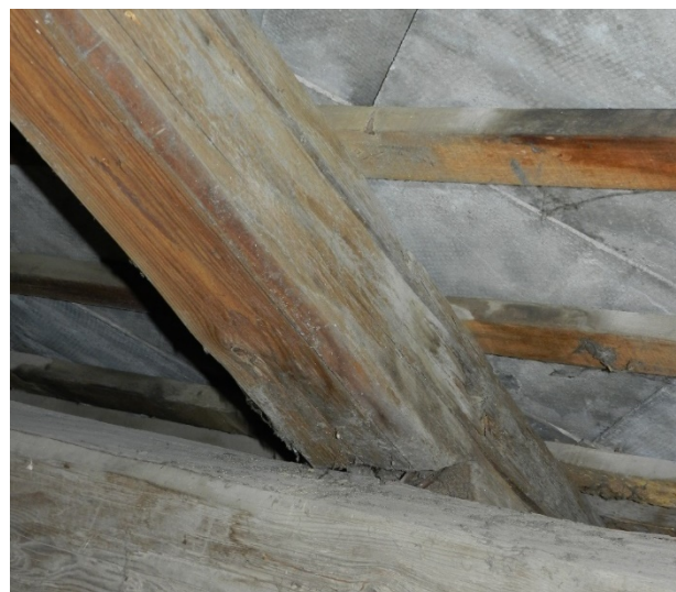
Figure 4. Loose connection of the rafter and lower purlin
