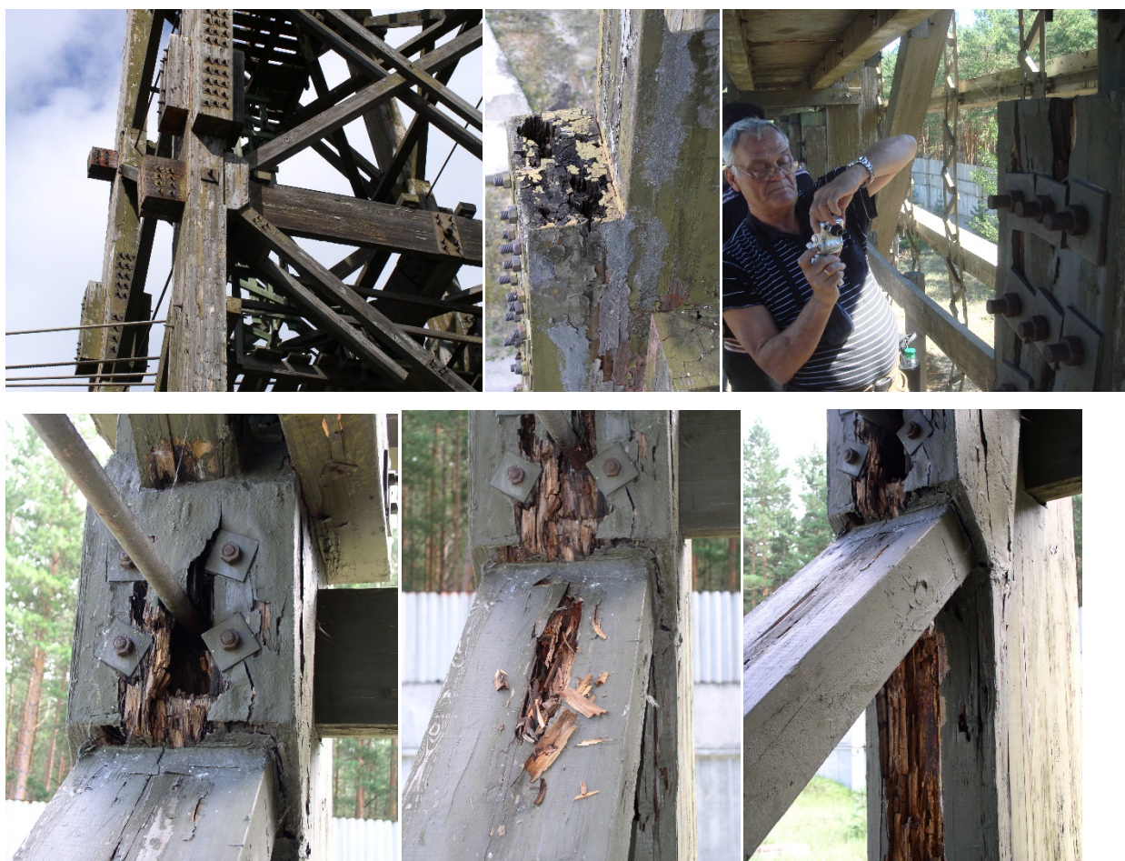
Figure 3. Cracks in structural elements and nodes during inspection in 2011
