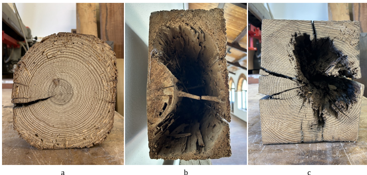
Figure 22. Different types of biotic decay in wooden beams (a) galleries and exit holes of anobiid and cerambycid beetles in the outer part, corresponding to the sapwood; (b) termite damage affecting almost the entire cross-section, except for the outer layer, the knots, and the pith; (c) fungal decay affecting the inner part.
