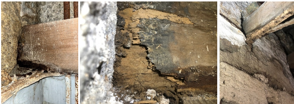
Figure 8. a) Beam of the chain that supports the ceiling of room S1.3 with damp and rot fungi; (b) Beam of the main beam of room S2.8 with rot fungi and beetle infestation; (c) Beam of the chain that supports the ceiling of room S2.2 with rot fungi and beetle infestation
