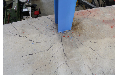
(b) Cracks in the concrete
