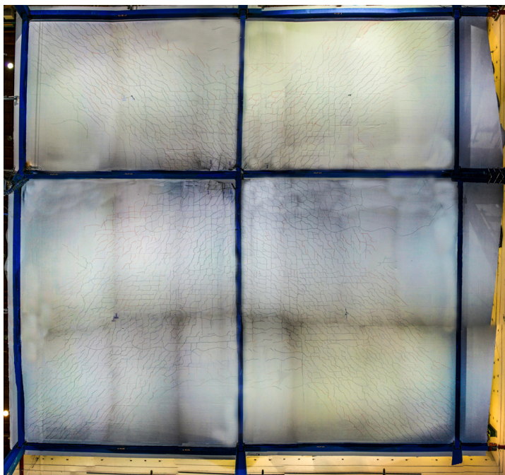
Figure 4.38: The cracking pattern on the bottom side of the slab - asymmetric sub-frame
