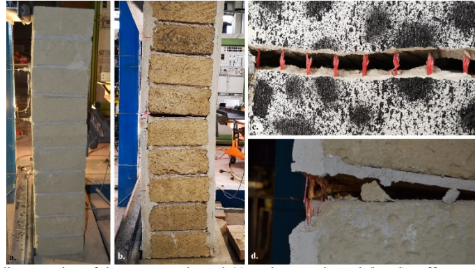
Fig. 16 – Failure modes of the unstrengthened (a) and strengthened (b,c,d) tuff masonry walls.
