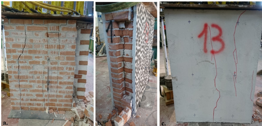
Fig. 9 – Failure modes of the unstrengthened (a) and strengthened (b,c) fired clay brick masonry walls.
