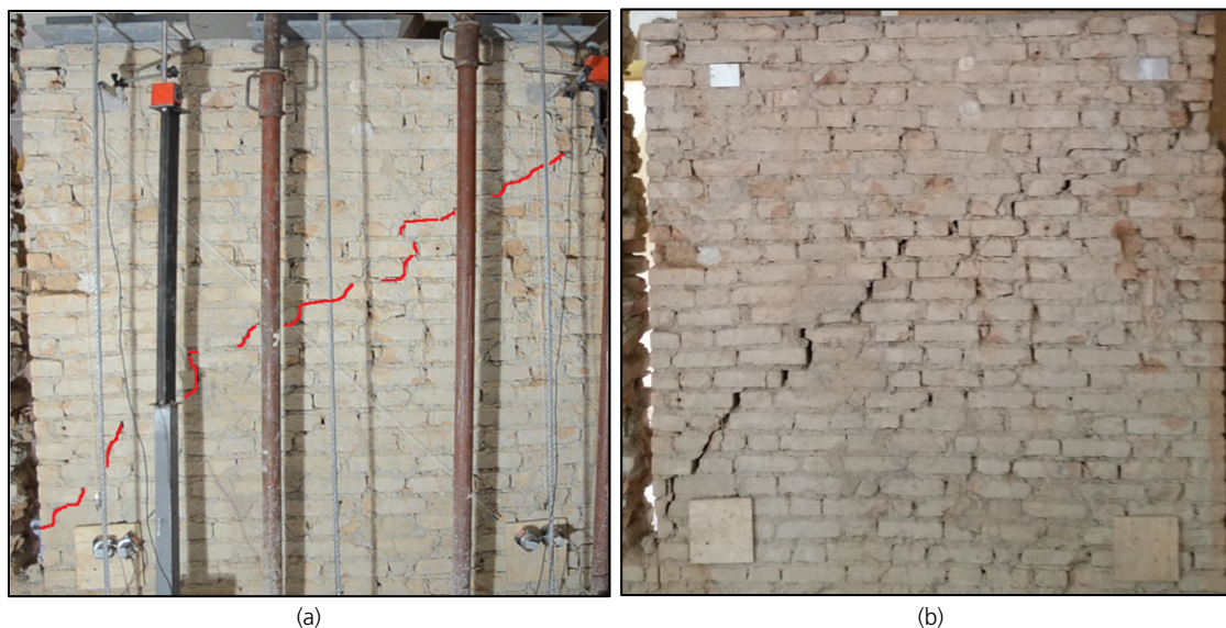
Figure 14. Damage to specimen R-3: (a) diagonal shear crack formation at peak loading; (b) crack pattern at the end of testing
