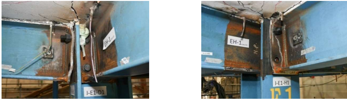
Fig. 22: The central node at collapse
