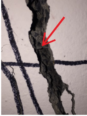
Fig. 31 Rupture of a stirrup due to tensile forces
