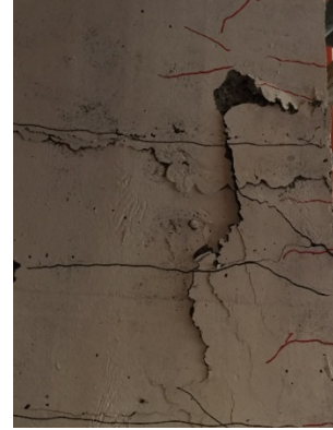
(b) Diaphragm failure in the right side
