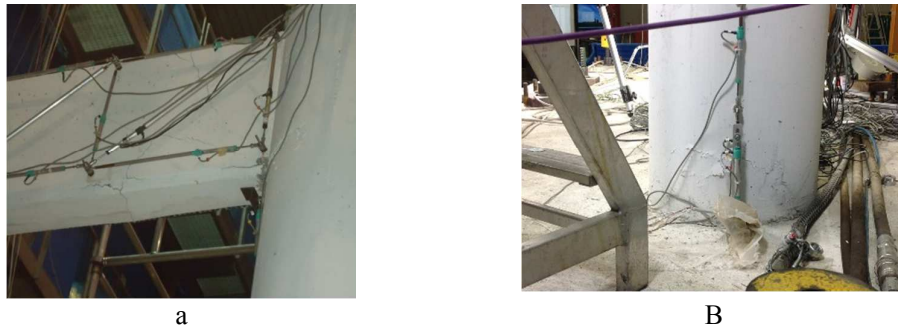
Figure 19. Close-up views of Pier #11: a) transverse beam; and b) left column, after HS k09.
